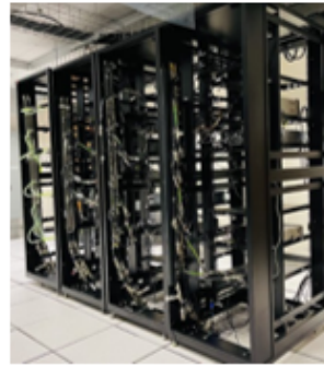
Liquid cooling rack system built from ground up.
